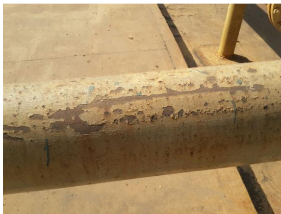
Example for pipe before cleaning
