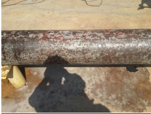
Example for pipe after cleaning with high pressure water and steel brush
